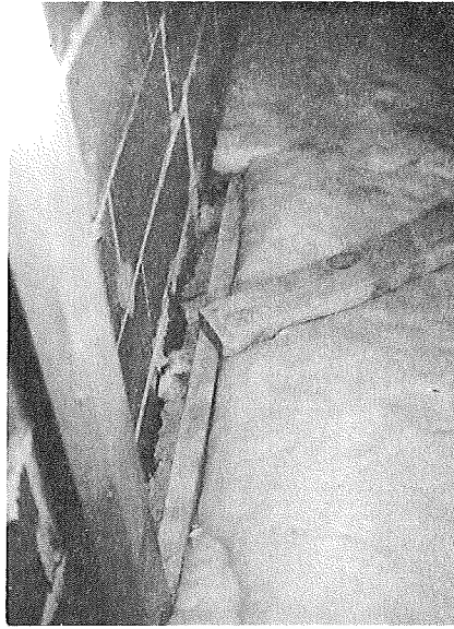
GAPS AT ATTIC FLOOR
