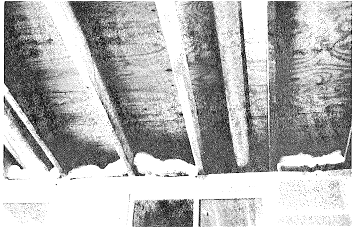
DUCTS PASSING INTO LIVING ROOM OVERHANG, CASUALLY INSULATED.
