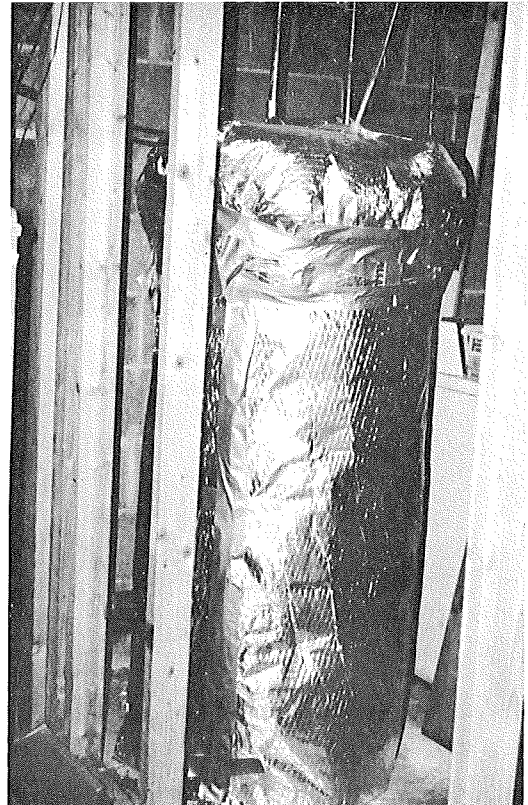
ELECTRIC HOT WATER HEATER FOLLOWING RETROFIT. WRAPPED IN FOIL BACKED R-7 INSULATION.
