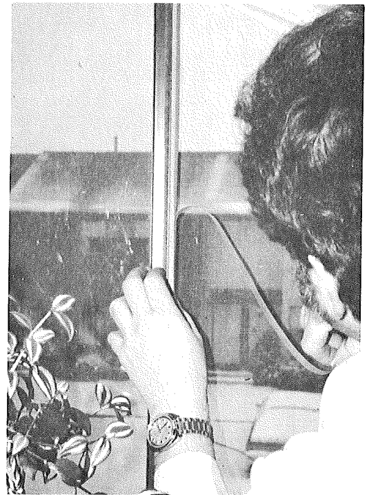
KENNETH GADSBY INSTALLS WEATHERSTRIPPING IN SLIDING PANEL OF PATIO DOOR, PART OF PRINCETON RETROFIT PACKAGE B.
