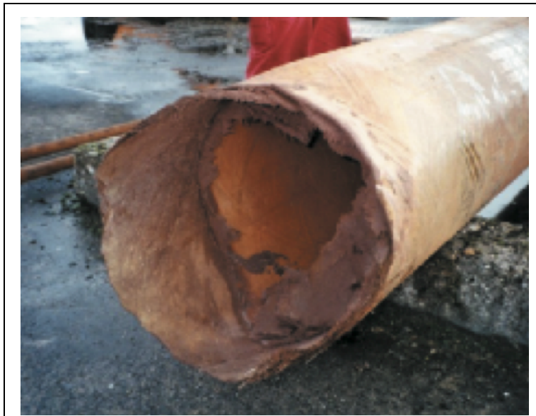
Figure 22 This photograph, from the Huntorf CAES facility in Germany, shows where the protective fiberglass-reinforced plastic tubing fractured. [35]
