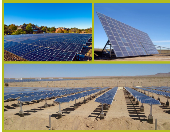
Figure 3.13 Panels in a fixed array at Eastern Mennonite University, Harrisonburg, Virginia (top left); with double-axis tracking in Toledo, Spain (top right); and with single-axis tracking in Xitianshan, China (bottom). Sources: Top left: https://upload.wikimedia.org/wikipedia/commons/c5/Eastern_Mennonite_University_Solar_Array.jpg Top right: https://upload.wikimedia.org/wikipedia/commons/8/8f/Seguidor2ejes.jpg Bottom: By Vinaykumar8687 - Own work, CC BY-SA 4.0, https://commons.wikimedia.org/w/index.php?curid=35401850 .
